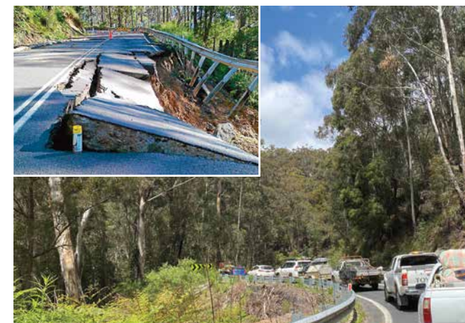
Figure 4-3: Damage and repairs on the highway at Brown Mountain. 7
